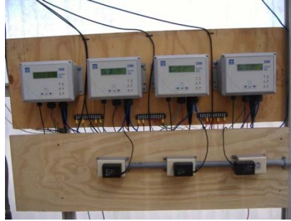
Figure 5: View of four units for DO monitoring
