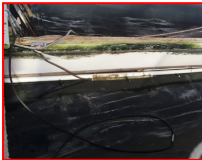
Figure 3: View of the center partition, the spray nozzles and one of the air diffusers
